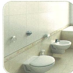
Toilet ISI standard fittings
